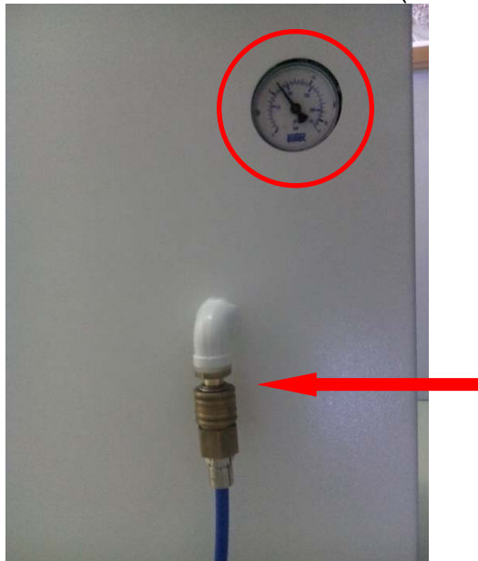
Picture 11. Compressed air connection
