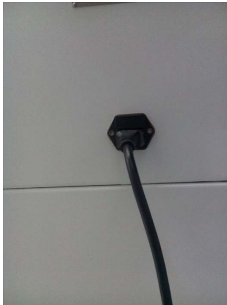
Picture 12. Power supply
