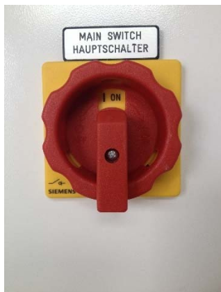
Picture 15. Main switch
